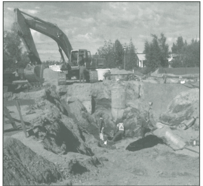
Figure 27. Underground utilities being replaced in sandy sediments beneath Forrest Drive during water and sewer upgrades in August 1997. GSC 1998-006 J
