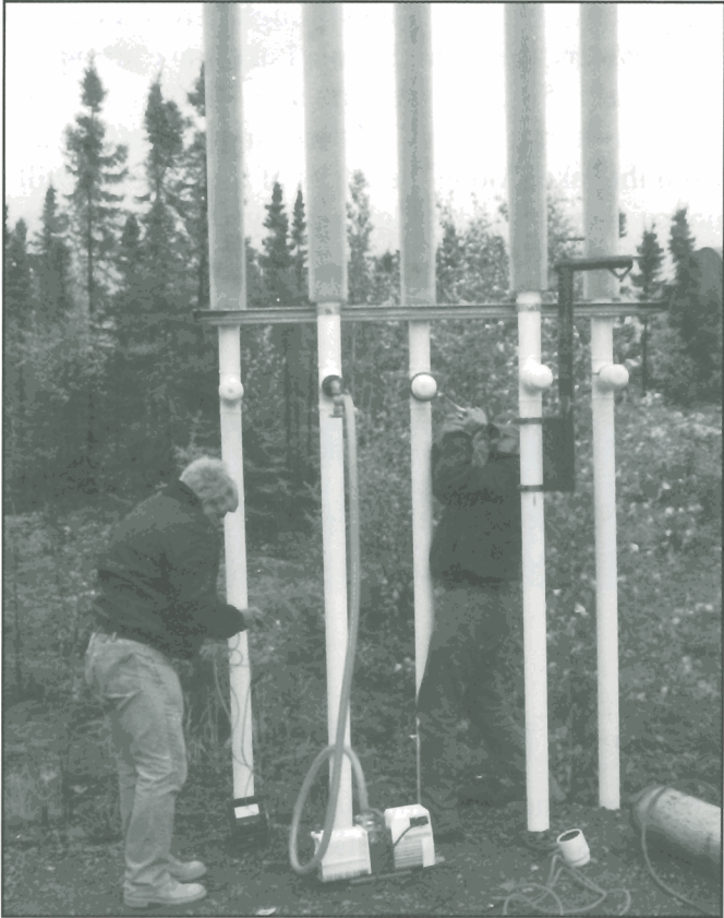
Figure 40. Stop 5 – Thermosyphons at the Legislative Assembly parking lot being charged with carbon dioxide (CO 2 ) gas. GSC 1998-006 P
