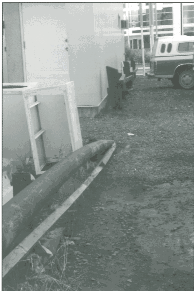
Figure 47. Stop 10 – Steel railing beside the northern corner of the Bowling Green building. The railing has been “swallowed” by the ground as the soil around the building has settled. A black wooden railing was put up beside the building after the steel railing had sunk into the ground. The wooden railing is now leaning towards the building because of the shifting soils. GSC 1998-006 U
