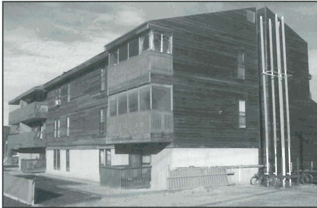
Figure 59. Stop 21 – Rockcliffe Apartments and thermosyphons used to stabilize the thawing of permafrost beneath the building. GSC 1998-006 CC
