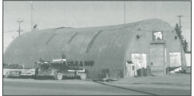
Figure 70. The Two-Way Enterprises building across from Fritz-Theil Park has undergone differential settlement due to thawing of permafrost. GSC 1998-006 JJ
