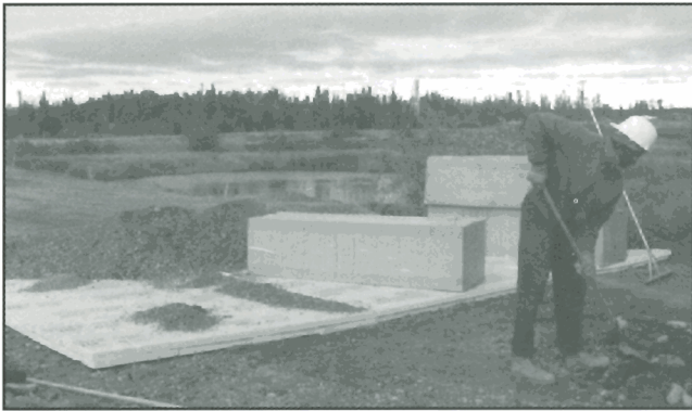
Figure 39. Insulation was placed beneath the road in order to preserve the permafrost. GSC 1998-006 O
