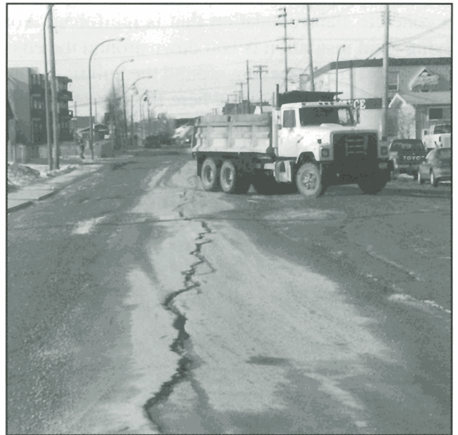
Figure 57. Frost heaving of silty soils beneath 52 Avenue caused the road to crack and bulge. GSC 1998-006 AA
