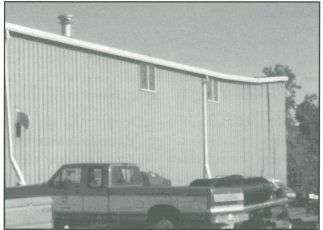
Figure 24. Frost jacking has lifted the right-hand corner of this building. GSC 1998-006 H
