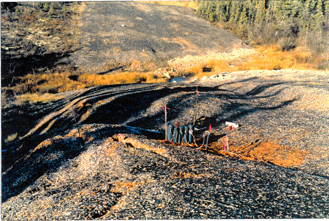
Plate 8. Slope 31A, Unnamed Creek South, KmP 84.5, Oct. 7, 1993. Northward view of slope with hot spot instrumentation. Note subsided hot area and ditchline, and tension cracks in the wood chips.
