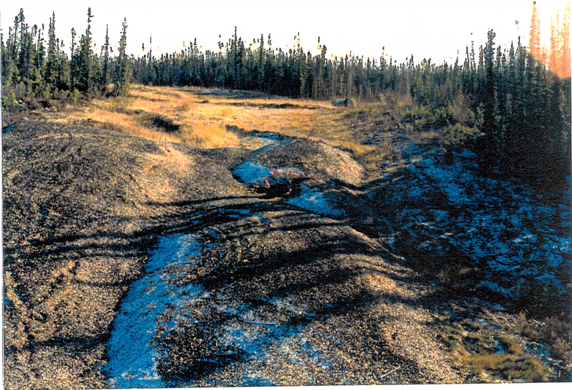
Plate 9. Slope 31A, Unnamed Creek South, KmP 84.5, Oct. 7, 1993. Aerial view towards the south of slope 31A with hot spot instrumentation.
