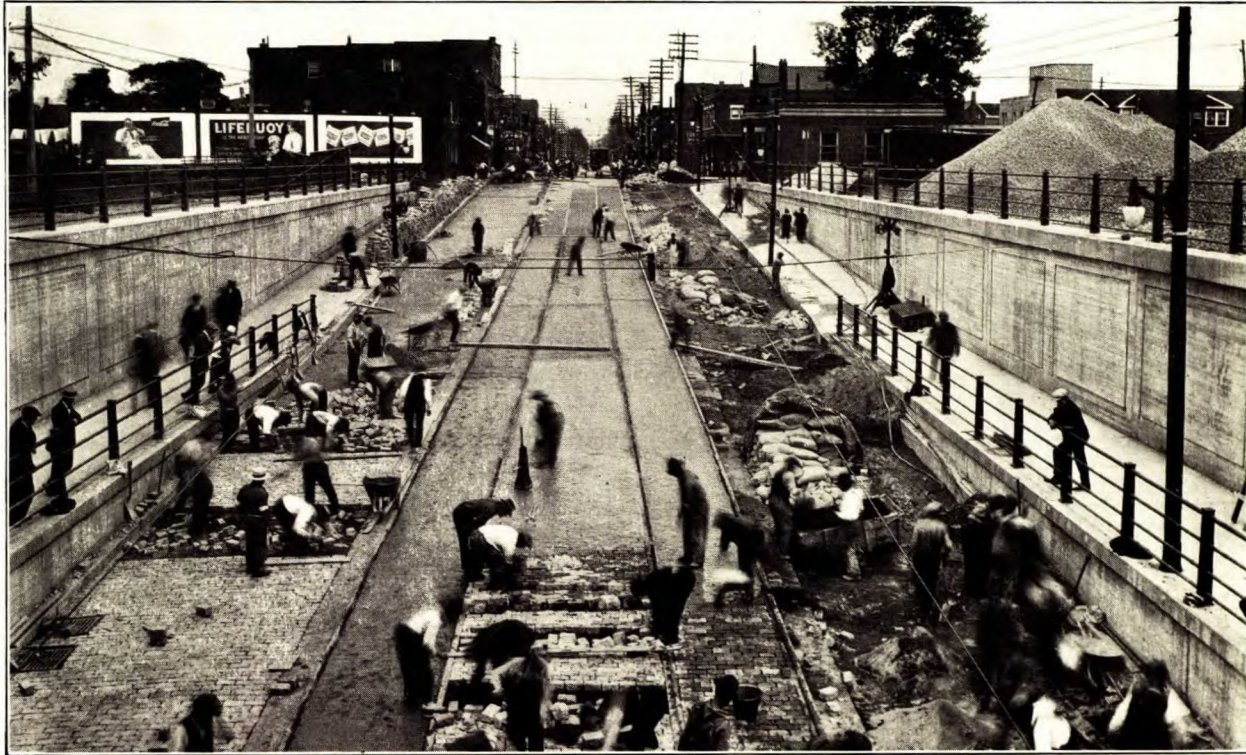
Bloor St. E., Toronto, from C.N.R. subway, showing method of laying granite paving blocks, and conditions under which the blocks have their greatest use.
