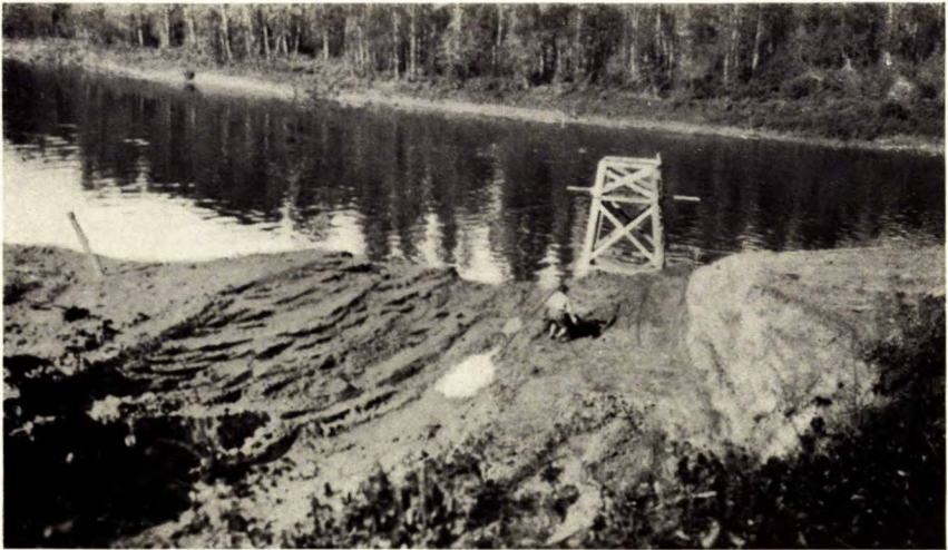
B. Commencing stripping of overburden; slip scraper and top of plank tower.
