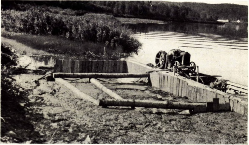
A. South end of crib wharf partly filled with material stripped from quarry site.
