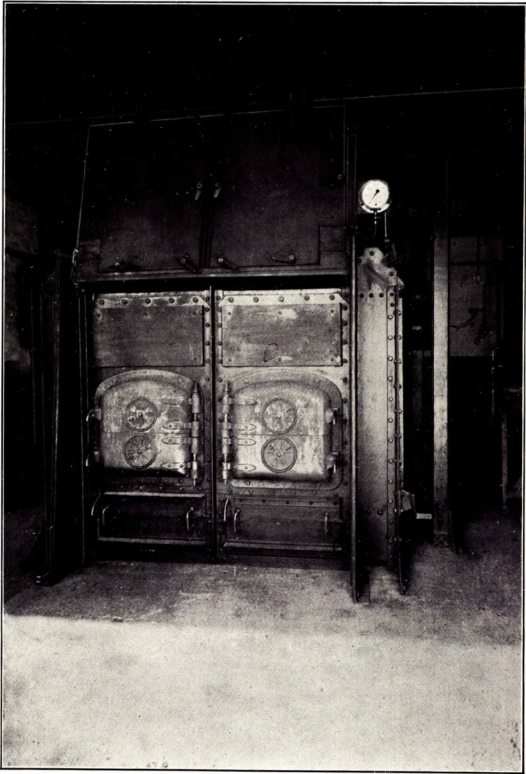
Fuel testing station: boiler room.
