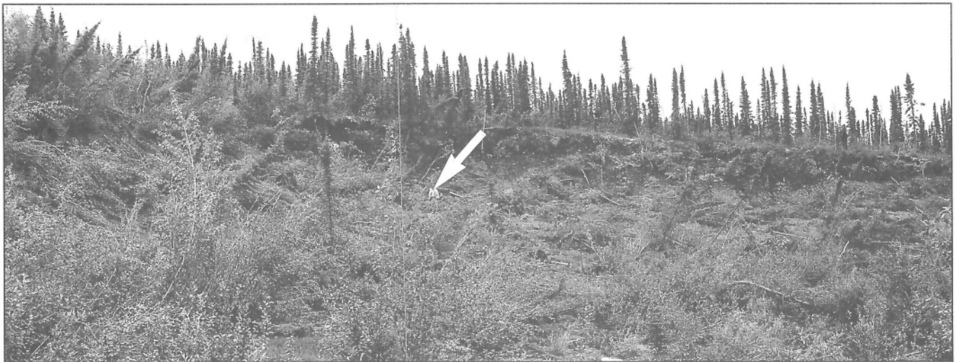
Figure 16. Active failure in the western part of element 3, June 1988. (The arrow indicates a man 1.7 m tall for scale.) GSC 1991-112
