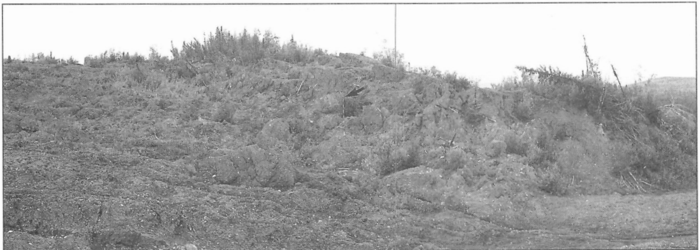
Figure 19. View looking southwest to west from the eastern side of the major failure of element 1 (C of Fig. 6). Landslide material is failing from the back (upslope side) of element 1 into the newly formed depression of element 7. (A 3.7 m ranging pole for scale indicated by the arrow.) GSC 1991-078B, 1991-078C
