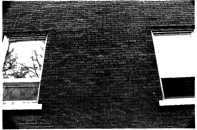
Diagonal cracks in brick wall of Notre-Dame Pavilion, Saint-François-d'Assise Hospital, Québec City
