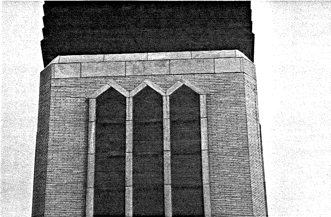
Figure 2.32 Cracking of masonry walls of bell tower.
