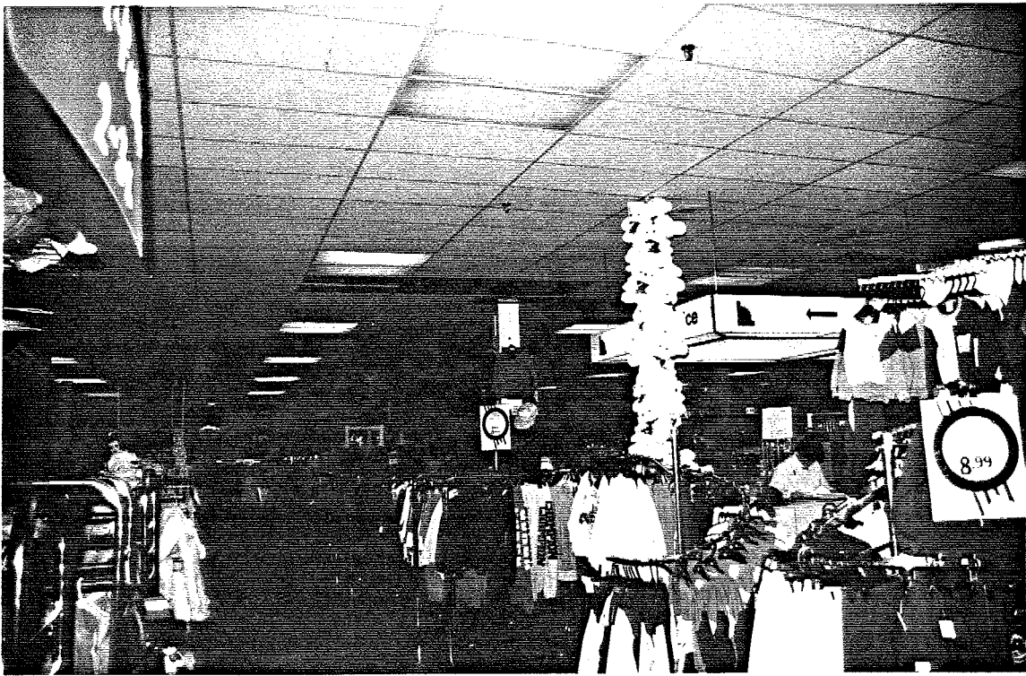
Figure 2.3 Damage to ceiling tiles in The Bay Store at Place du Royaume Shopping Plaza.
