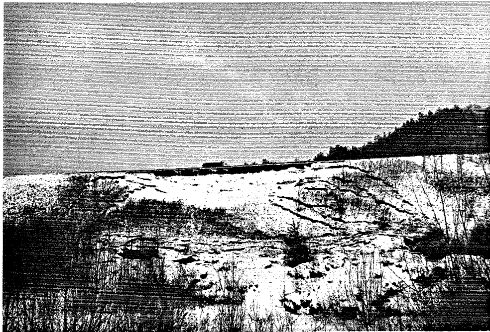
Figure 6.2 Overall view of embankment failure.
