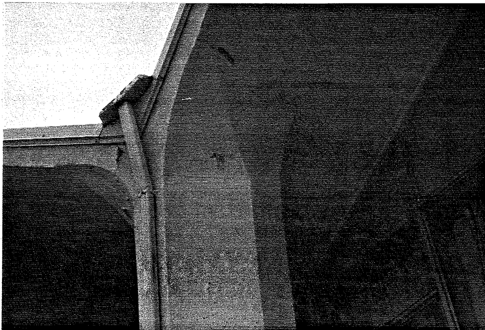
Figure 3.21 Cracking of column and roof slab.
