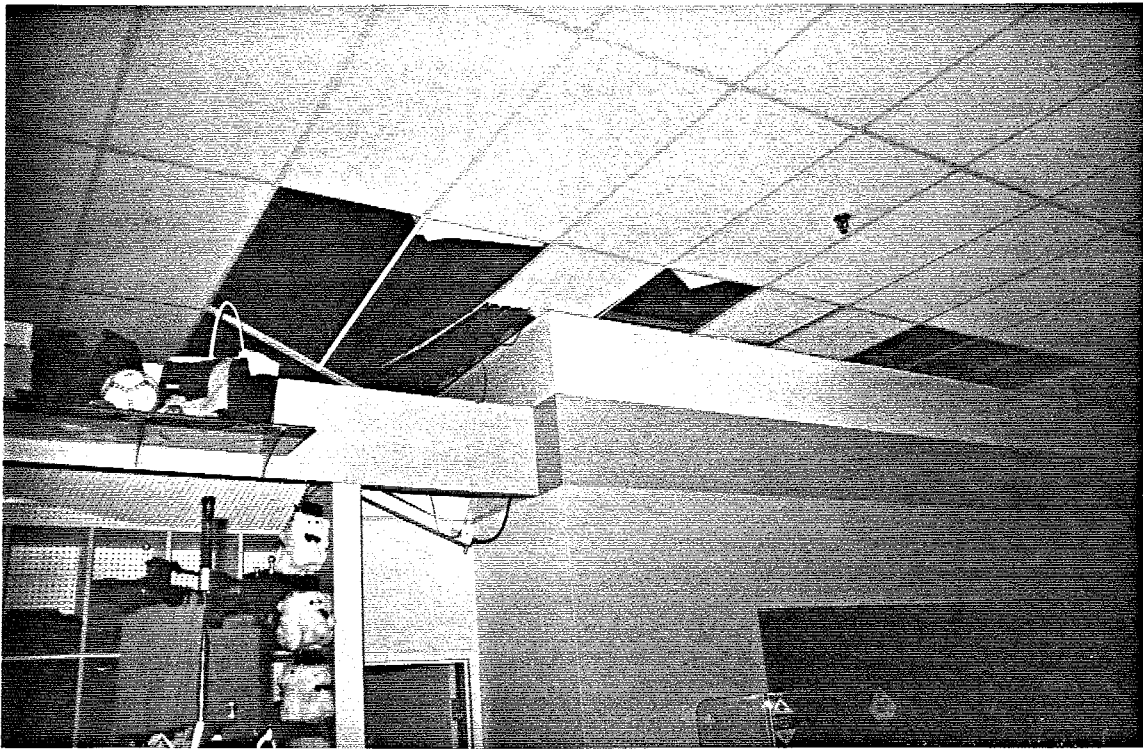
Figure 2.5 Damaged ceiling tiles due to fallen masonry blocks in The Bay store.
