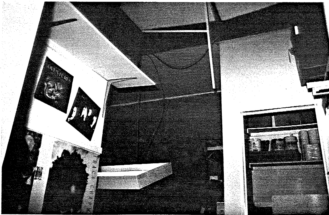
Figure 2.8 Damage to light fixture in Kébec Disque store due to loss of support.
