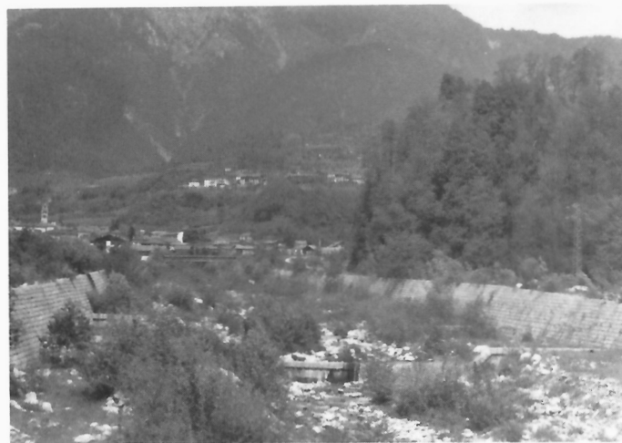
Figure 277: Reconstructed masonry-lined channel of the Chiappena Torrent below Strigno; note armoured sills defining the normal discharge section of the torrent. (GSC 204170-B)
