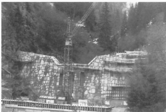
Figure 165: Protective dam under construction above the apex of the Axams cone; note vertical slits in the dam which allow selective discharge of normal bed-load and minor debris flows. (GSC 204167-U)
