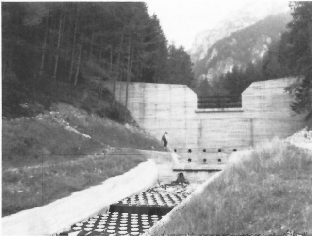
Figure 71: Protective steel-concrete dam at the mouth of Val Bonetta. The lined channel permits nondestructive discharge of small debris floods spilling over from major flows that would be retained behind the structure. Note drainage bores at the base and selective discharge section ('filter dam') at the crest. (GSC 204165-Y)
