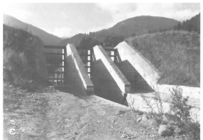
Figure 17: Examples of protective debris retention dams: a) masonry-lined steel concrete dam with vertical selective discharge slits under construction (near Innsbruck, Austria) (GSC 204165-E); b) steel-concrete dam; note drains in the lower half and selective discharge section of steel beams above (near Caoria, Italy) (GSC 204165-F); c) buttressed selective discharge section of an earth-rockfill dam (near Innsbruck, Austria) (GSC 204165-G).
