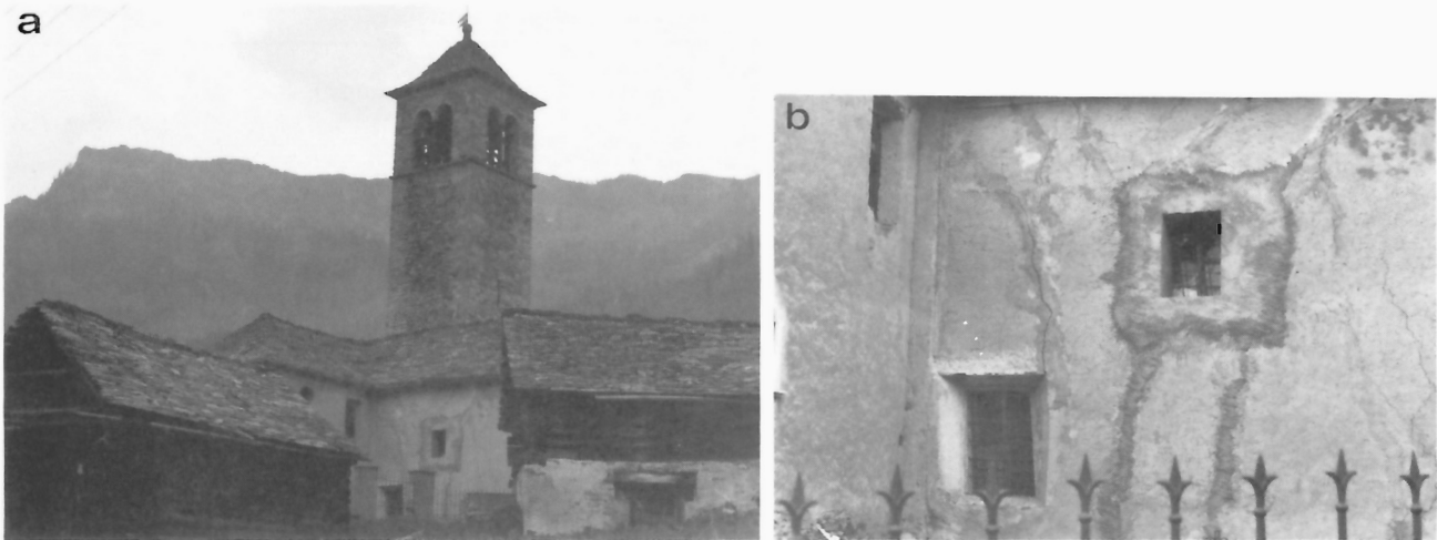
Figure 213: a) The old church of Campo which during the last century has shifted at least 15 m horizontally (GSC 204168-V). b) Close-up view of the cracked and distorted church wall (GSC 204168-W).
