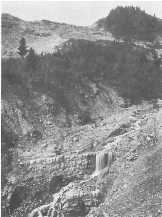
Figure 209: Slumping bedrock embankments along the Nolla channel as seen at the turn of the century; note shifted and partly crushed masonry check dams (from Salis, 1914).
