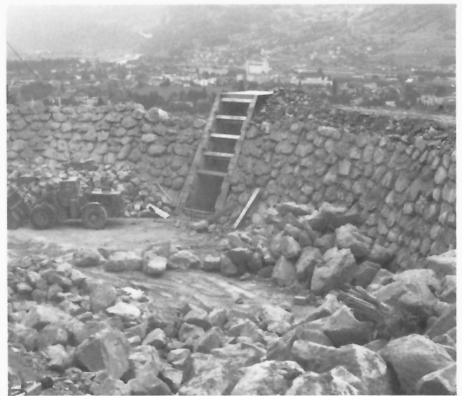
Figure 224: Protective dam against debris avalanches under construction near Altdorf; note stone block armour and discharge section designed to drain water from complex debris-snow avalanches. (GSC 204169-D)
