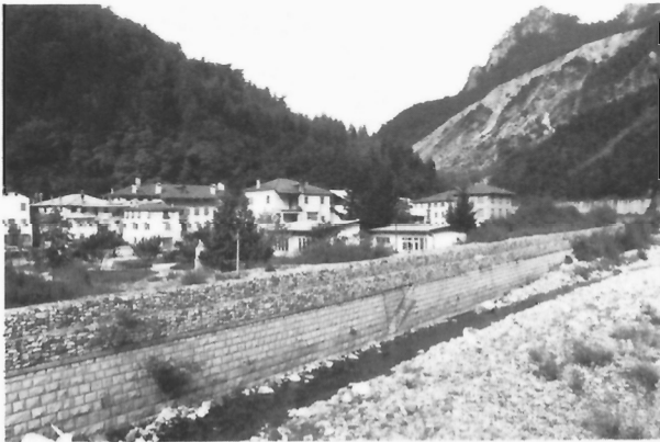
Figure 183: Masonry and gabion dyke separating the town of Perarolo from the channel of the Bòite Torrent; unstable bedrock slopes upstream from Perarolo in the background. (GSC 204168-D)
