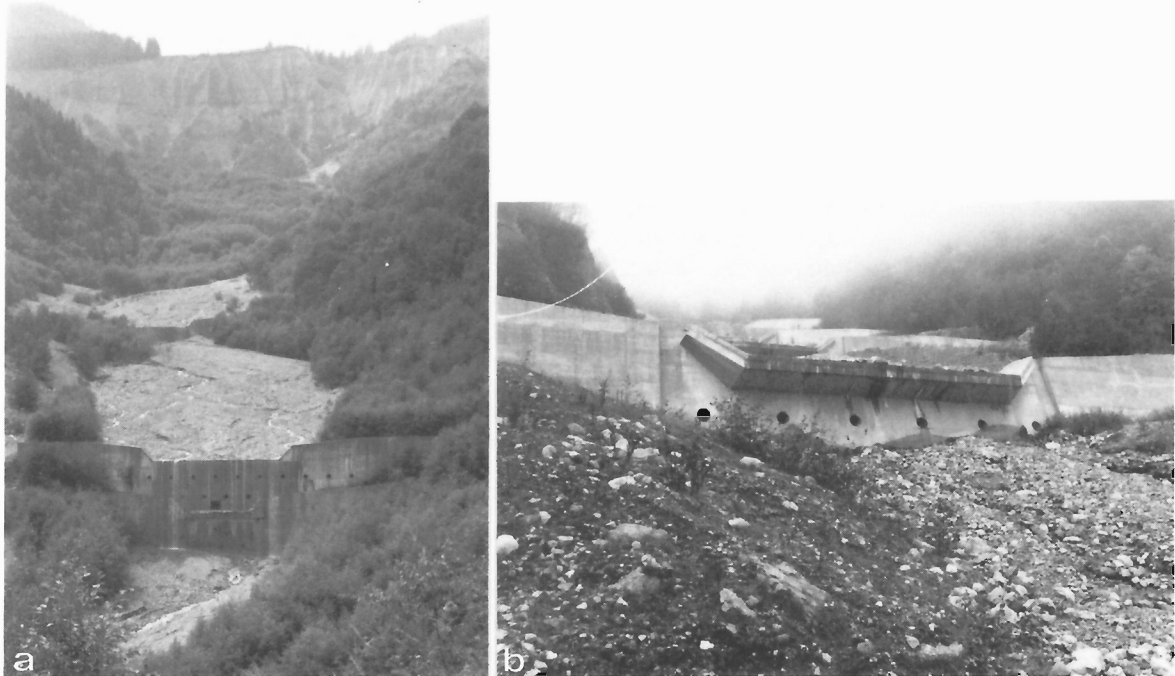
Figure 174: Two views of the large check dams along the Schesa Torrent below the erosional bowl of the Schesatobel: a) check dams confining the braided channel of the Schesa Torrent to the centre of the valley thus preventing lateral scour (GSC 204167-Y); b) steel-concrete check dam with an armoured carapace which minimizes damage to the structure from minor debris flows (GSC 204167-Z).
