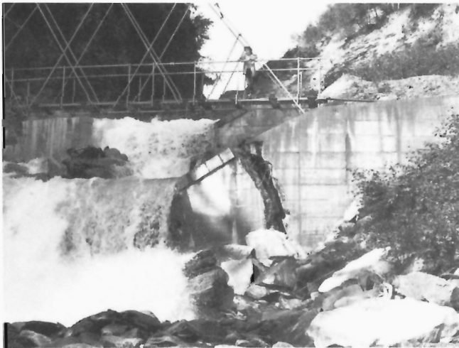
Figure 280: Check dams across the Gradenbach Torrent; note damage to the abutments of the check dams caused by lateral pressure from the toe zone of the sagging Eggerwiesenkopf slope. (GSC 204170-C)
