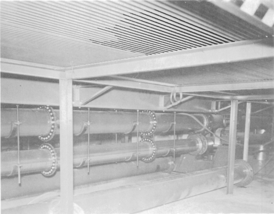
Figure 6. Transparent acrylic sections in return pipes beneath main channel. GSC photo 201625-E
