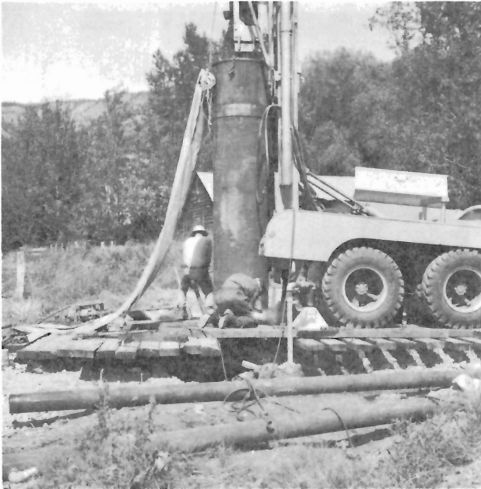
Figure 9. Welding 30 inch casing joint. Driving head in position on casing in preparation for driving casing with the diesel hammer. GSC 125293.
