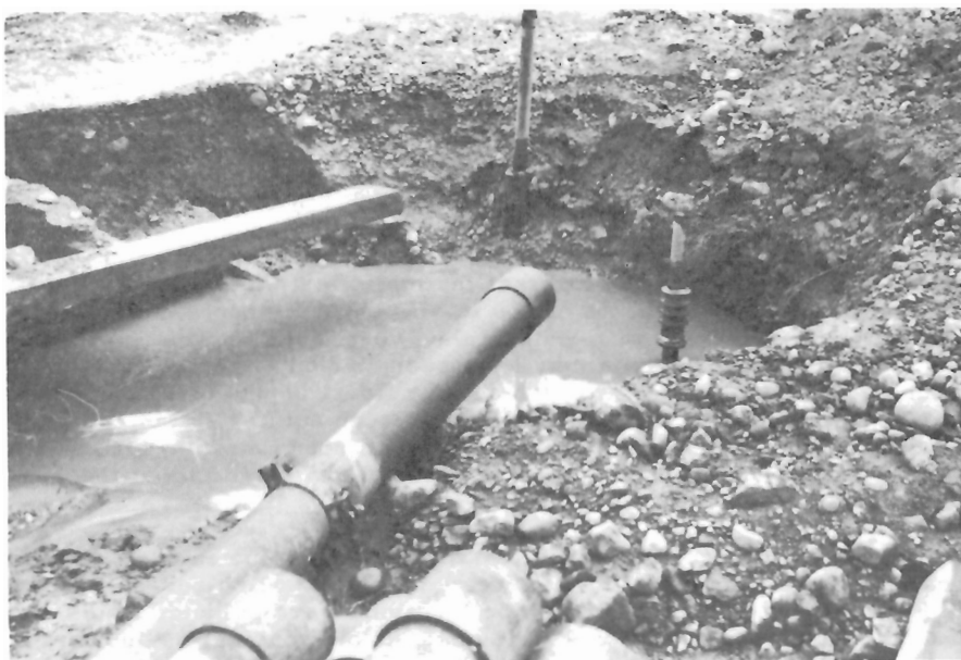
Figure 4. Initial stage of collapse at well site. August 1966. Note wiper plug used as casing seal on 2 inch pipe. GSC 118665.
